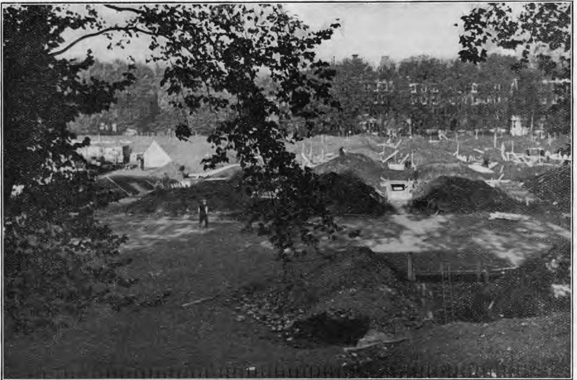
A view of Fields to-day showing the extensive alterations imposed by the Government's Air Raid Precautions.
