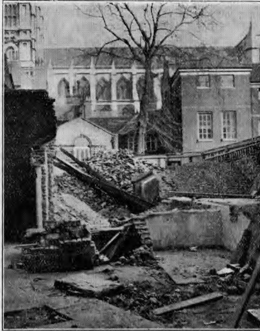
The Demolition of the Fives Courts in Yard; part of the plans for preparing No. 17, Dean's Yard for use as a School Building.
